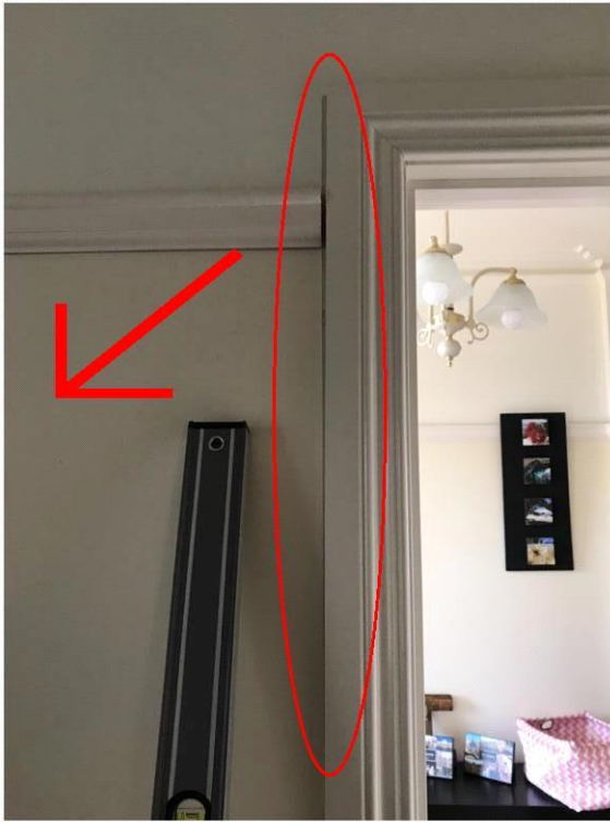
slight separation noted to bed 1 wall
