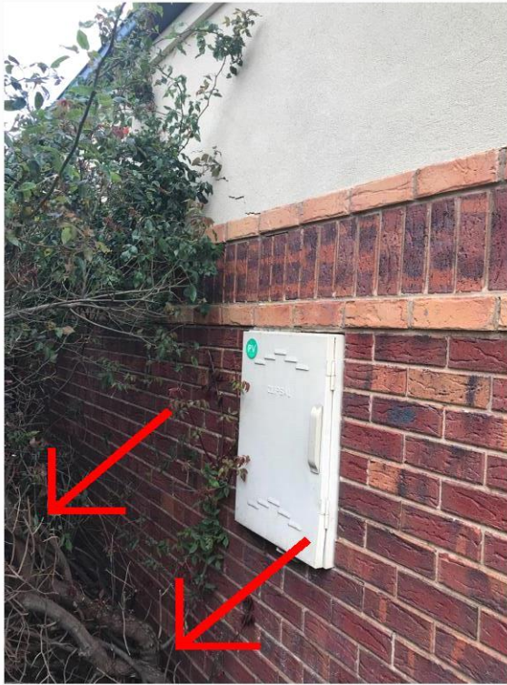
subsidence noted to strip footing
