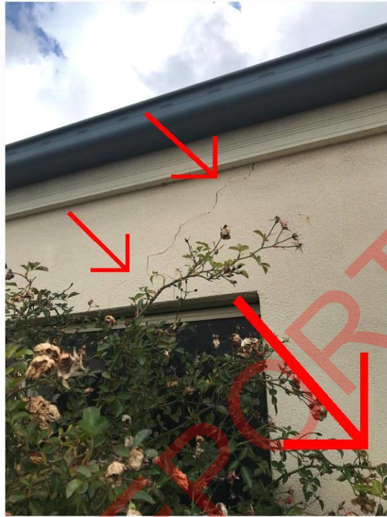
movement cracking viewed to rear garage
