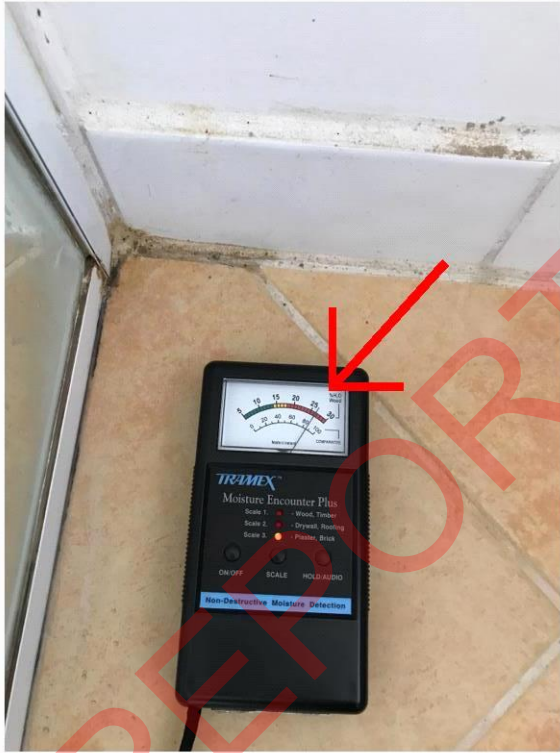
high moisture recorded to floor tile
