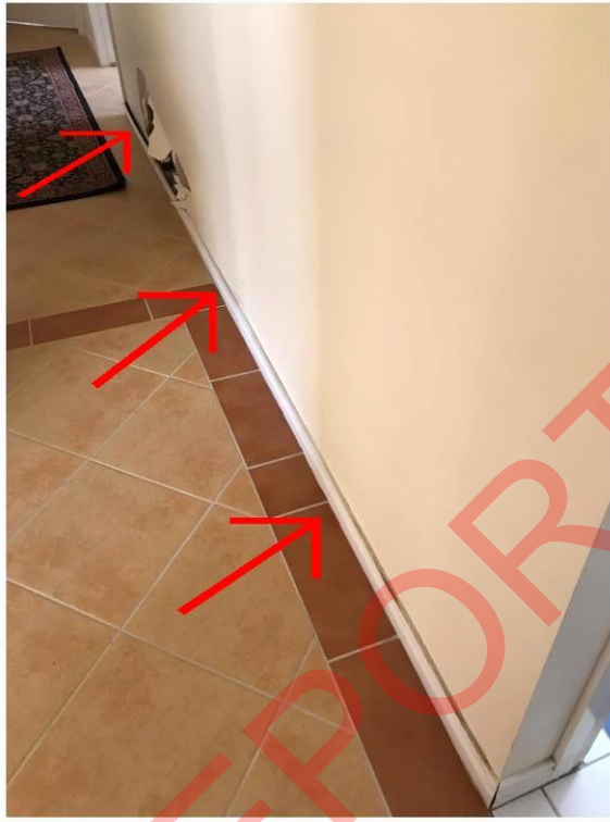
visible shower leak defects noted
