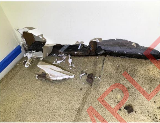
water staining viewed & strong odour
