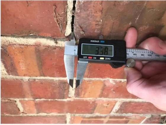
measured garage wall crack example
