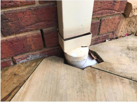
DP not connected to PVC adaptor
