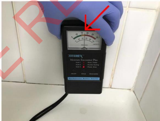
high moisture recorded to recess wall tile
