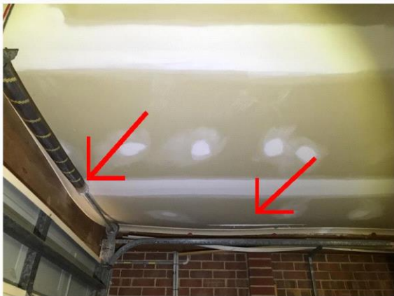
visible sagging of ceiling example
