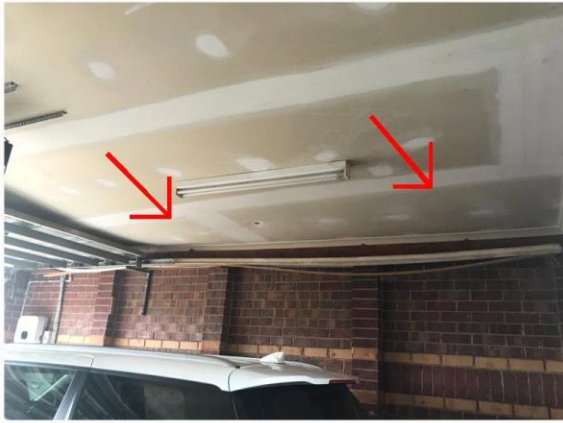
visible sagging of ceiling example
