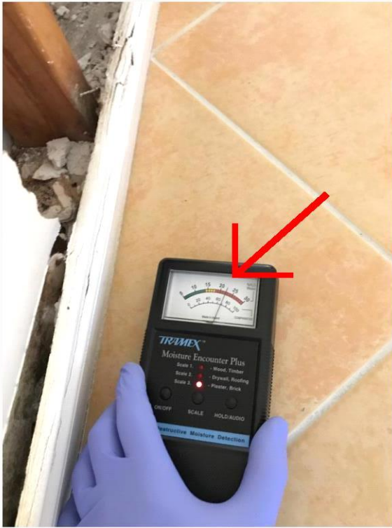
high moisture to hall floor from shwr leak
