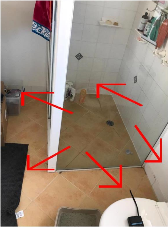
water spread from walk-in shower active
