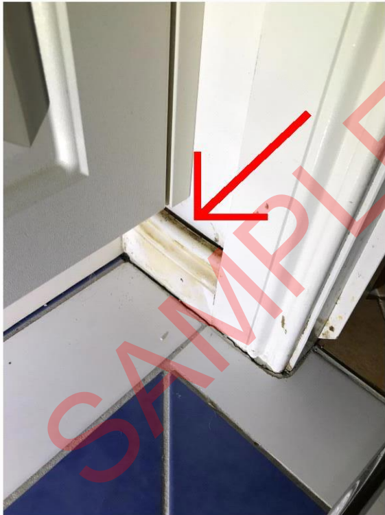
visible shower leak defects noted (laundry
