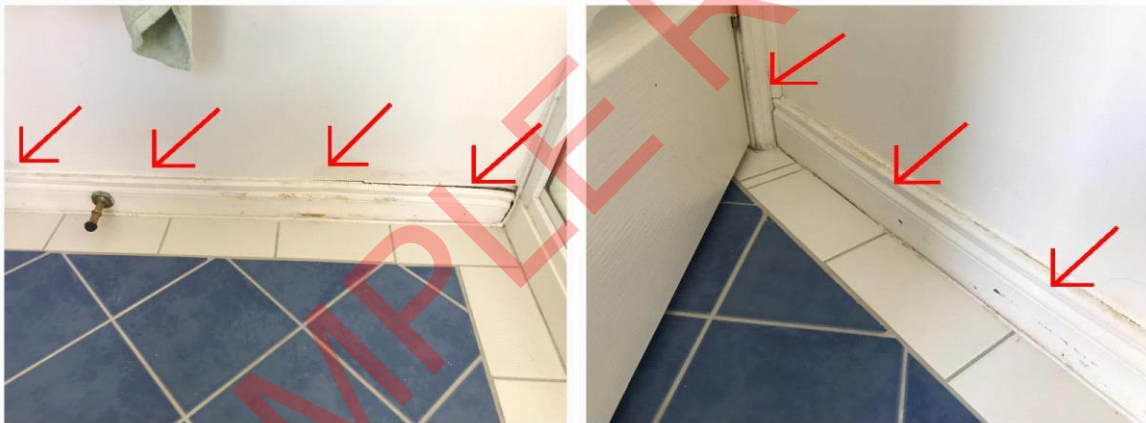
visible shower leak defects noted
