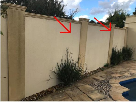
leaning noted | heavy cladding
