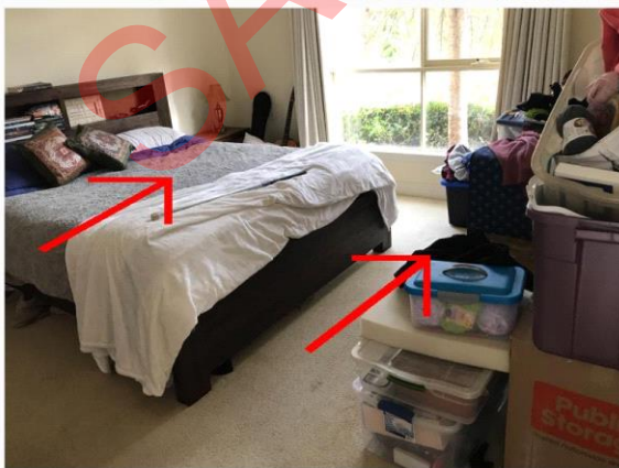
area of level deviation within bed 1
