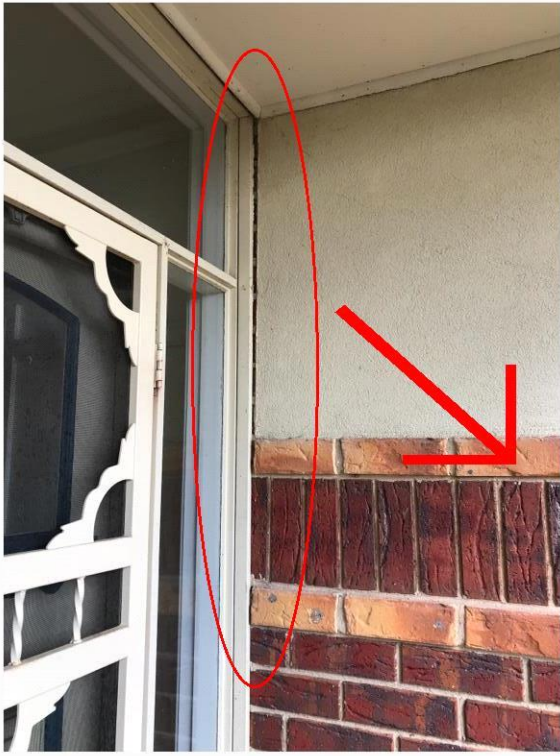
separation noted to wall|drop toward front
