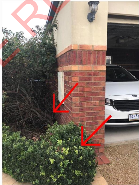
subsidence noted to strip footing
