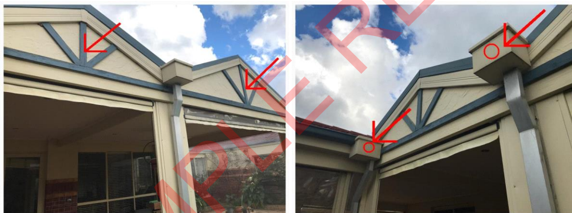
paint protection required example
