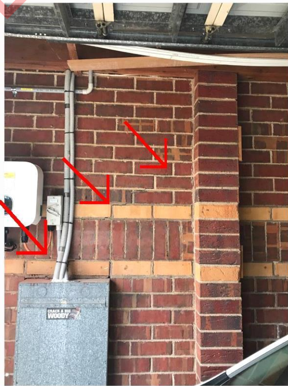
movement cracking viewed to garage wall
