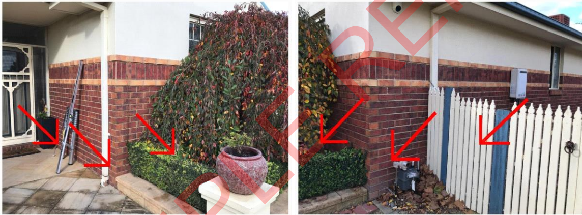
slab subsidence noted to main bedroom
