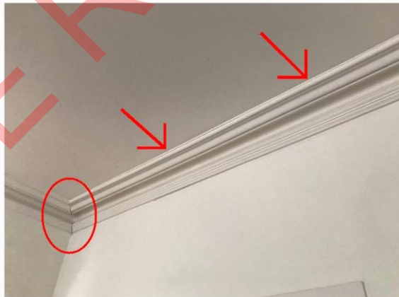
settlement cracking viewed (main bed)
