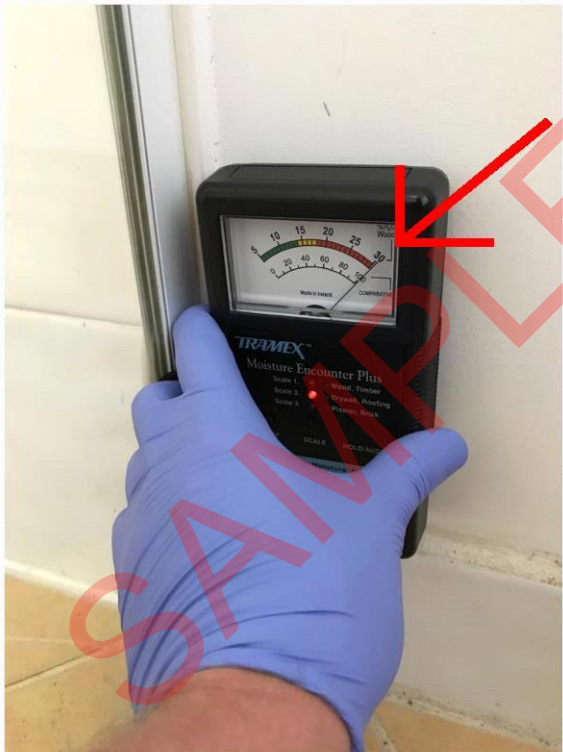
high moisture recorded to wall lining (RS)
