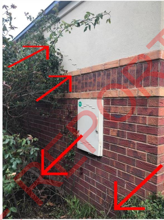
movement cracking viewed to garage wall
