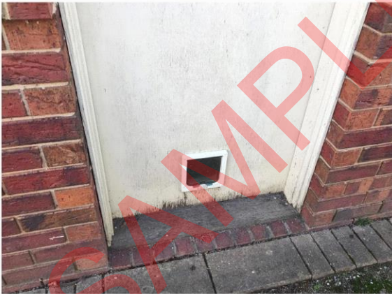
weathering to exposed door example
