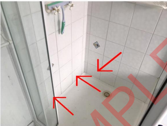
high moisture recorded to recess walls
