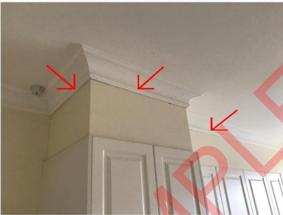
minor settlement cracking viewed (kitchen)
