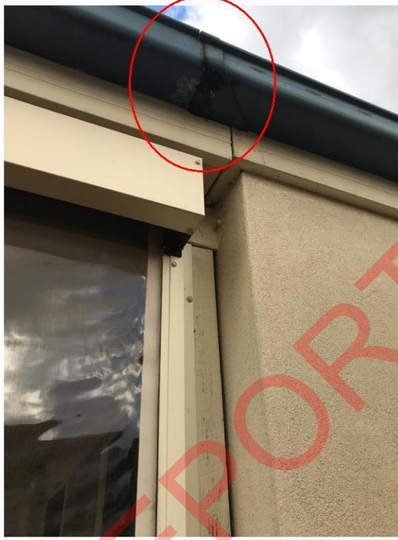
make good / rework gutter joint leaks
