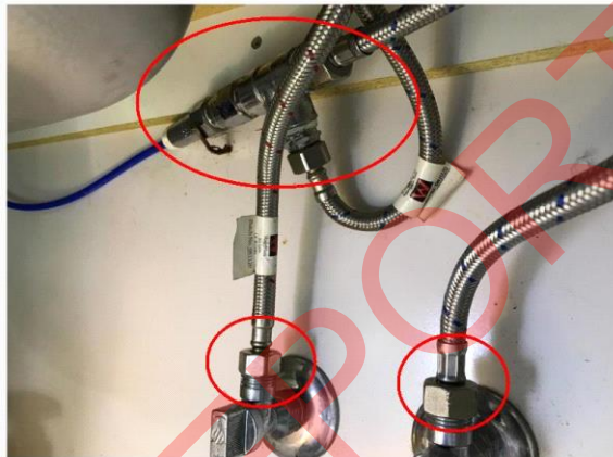
have plumbing connections assessed
