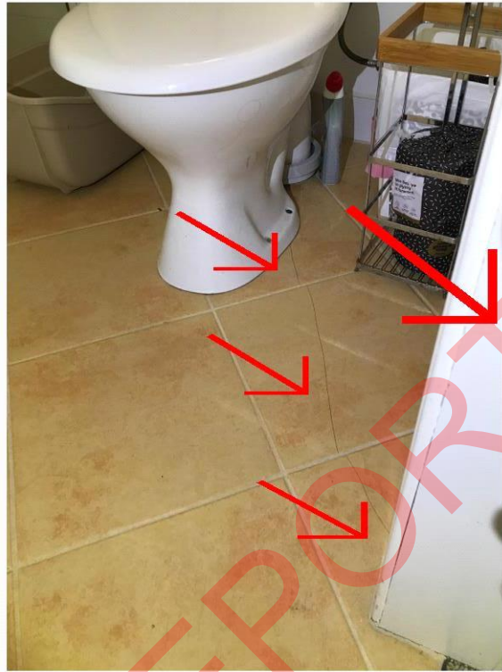
tile cracking from slab movement viewed
