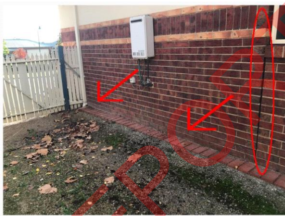
separation noted to wall|drop toward front
