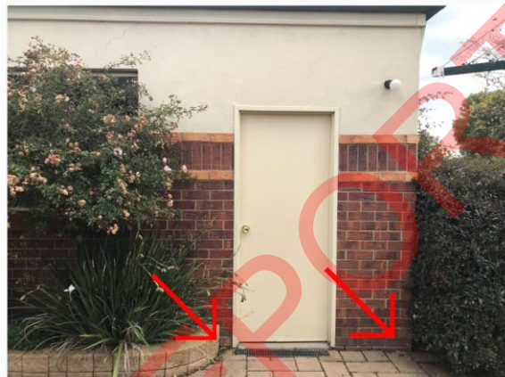
subsidence noted to strip footing
