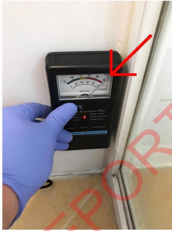
high moisture recorded to wall lining (LS)
