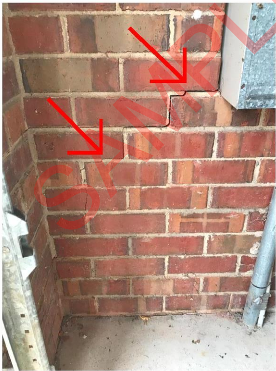
movement cracking viewed to garage wall
