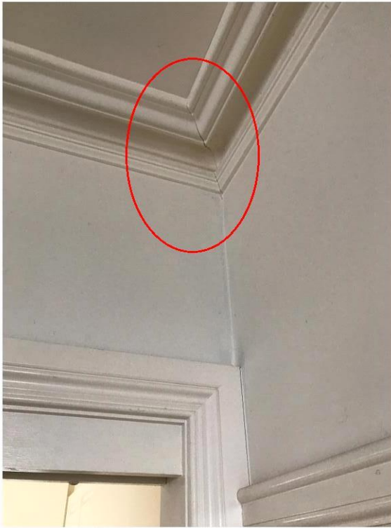
minor settlement cracking viewed (hall)
