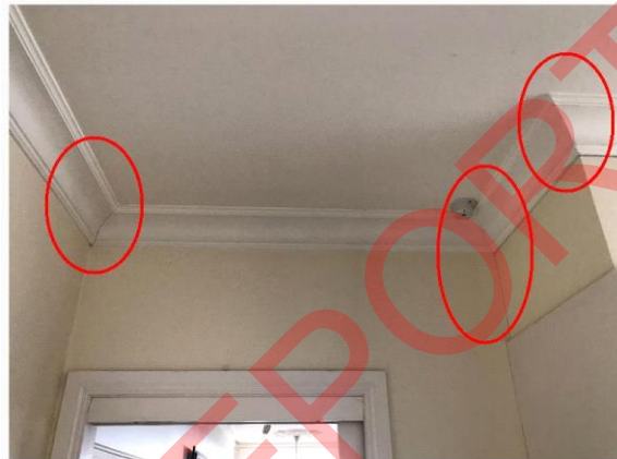
minor settlement cracking viewed (kitchen)
