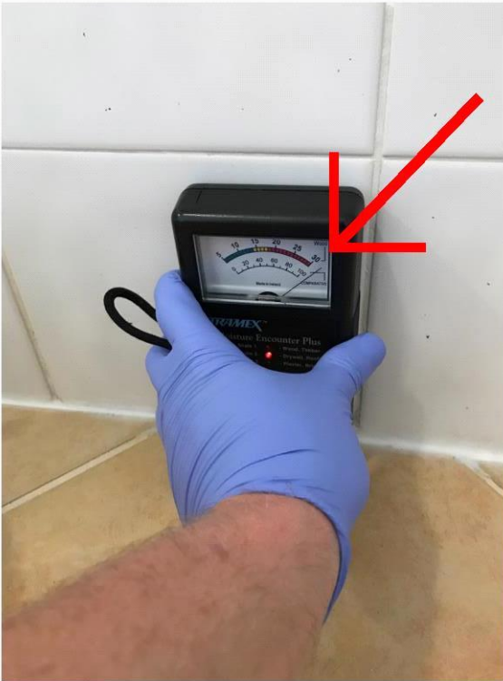
high moisture recorded to recess wall
