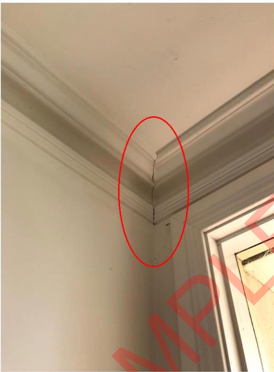
settlement cracking viewed (entry)
