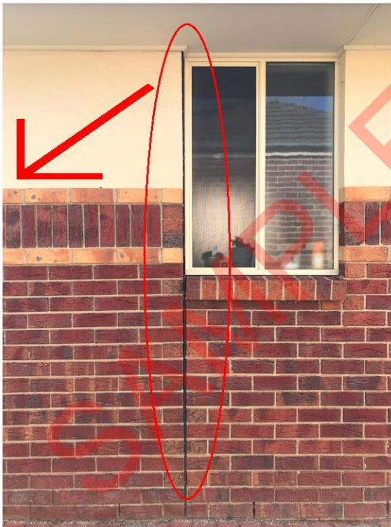
separation noted to wall|drop toward front
