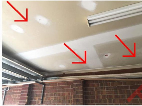
visible sagging of ceiling example
