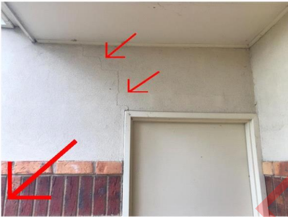
movement cracking viewed to garage wall
