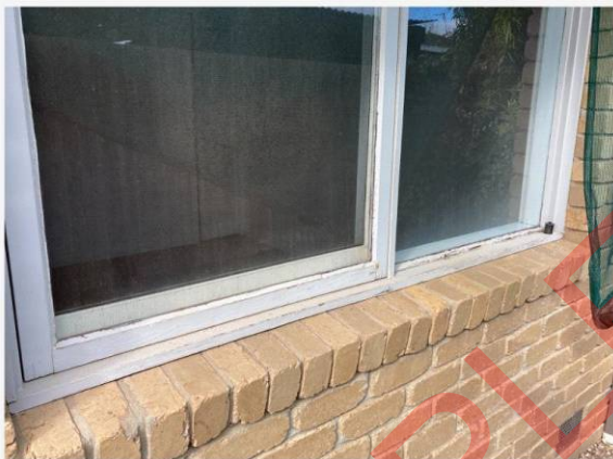
weathering/paint peel/minor decay noted
