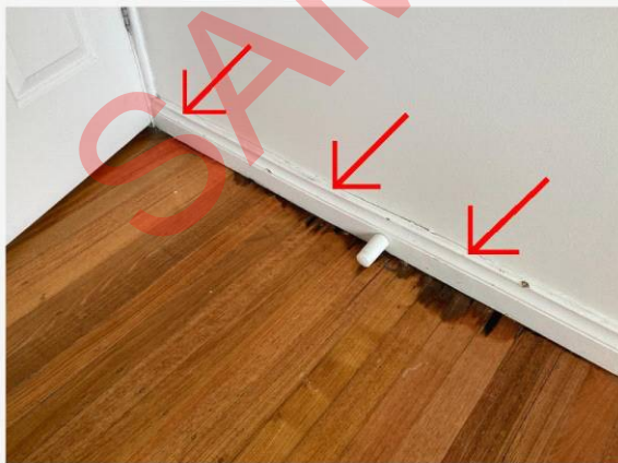
water spread / breach noted
