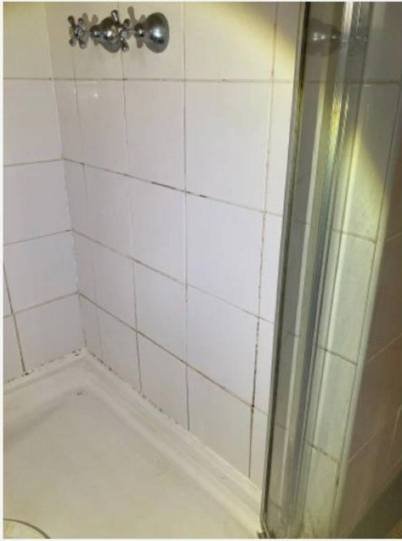
waterproofing defects visible
