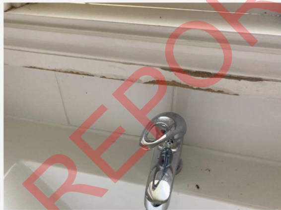
water splash damage to MDF trim
