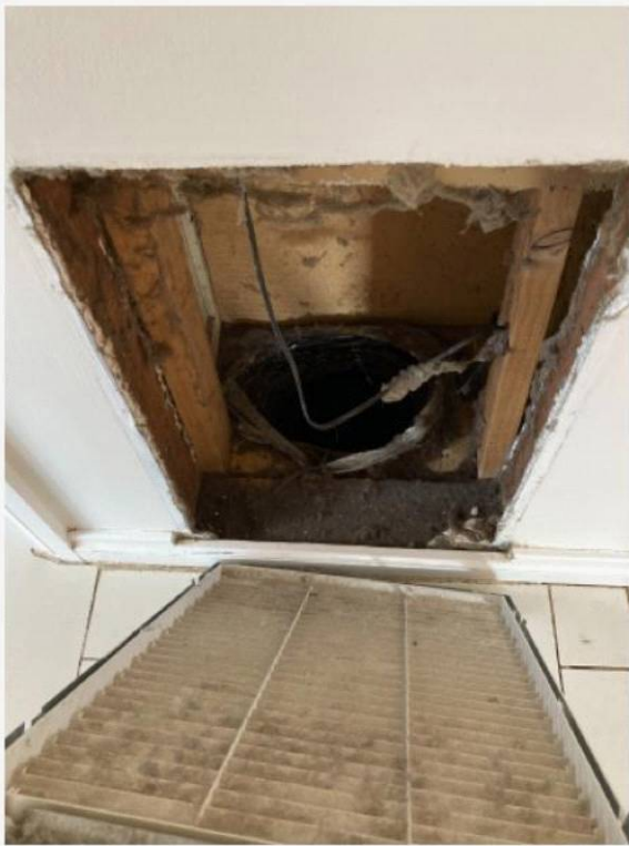
recommend filter to return grille
