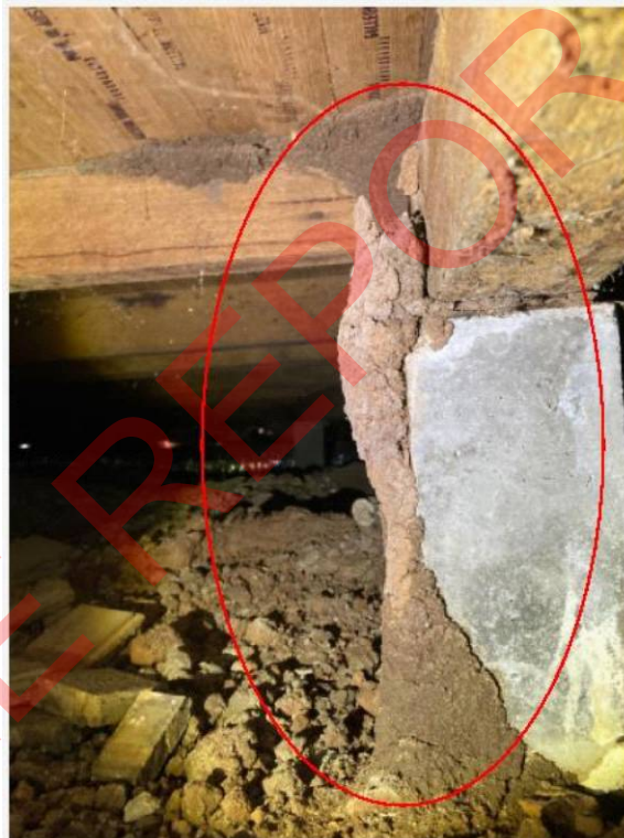
termite mud lead noted below entry/lounge
