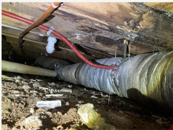
significant shower leak defects noted
