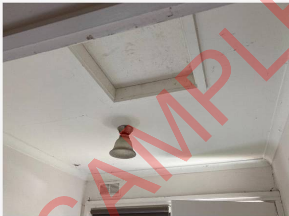
sagging/drop in ceiling noted example
