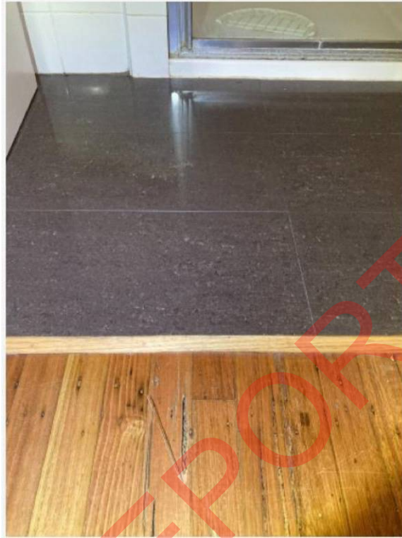
termite attack damage viewed to flooring
