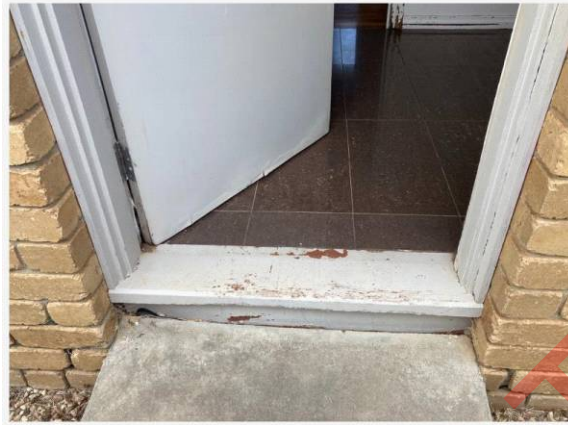
water entry/weathering through door likely
