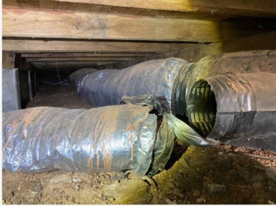
duct disconnected| re-tape
