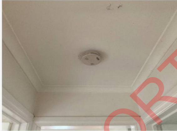
smoke detector fitted example
