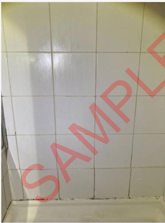
waterproofing defects visible
