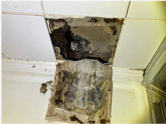
water breach noted
