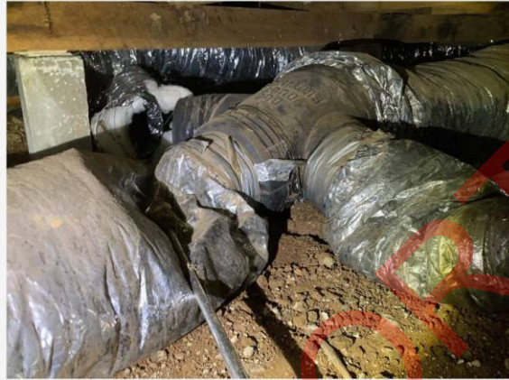
duct squashed| replace affected section
