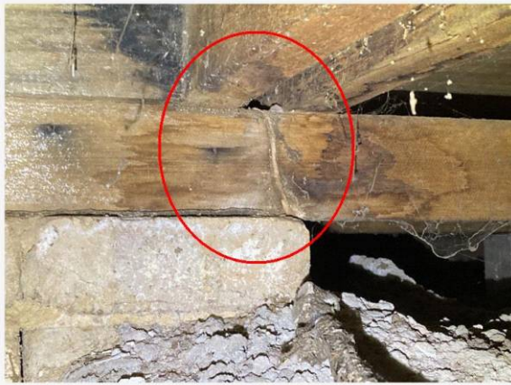
termite mud lead noted below entry
