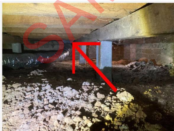
termite attack damage through lounge
