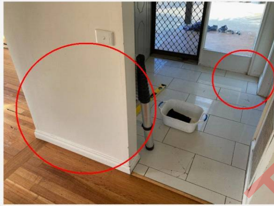
areas of termite attack entry noted below
