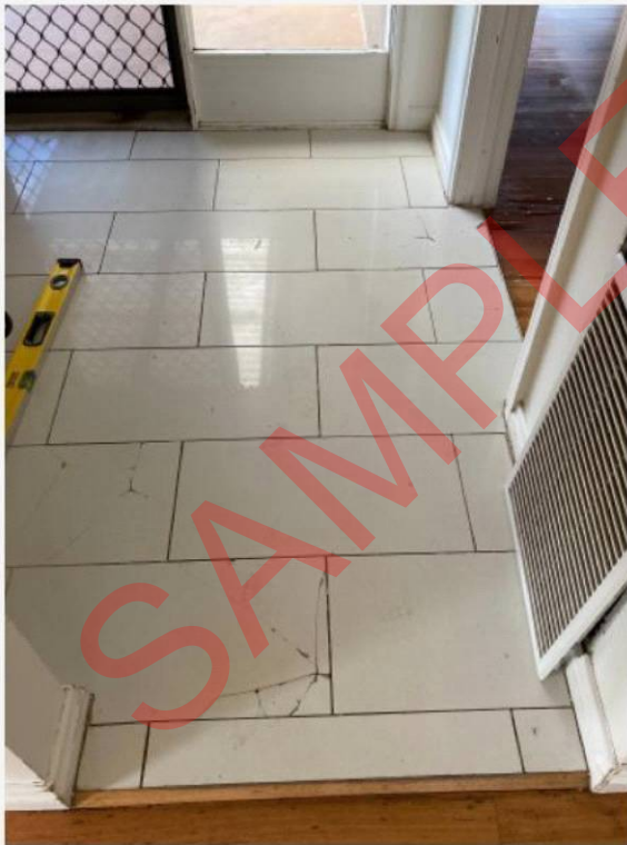
tile cracking from substrate damage
