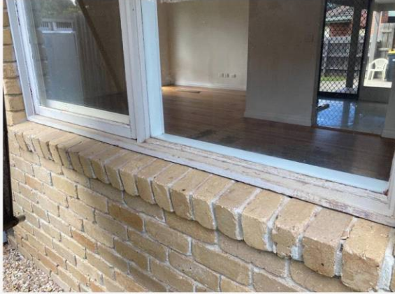
weathering/paint peel/minor decay noted
