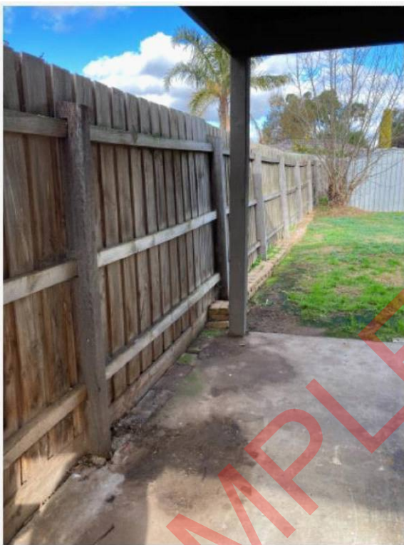
LHS fence leaning but stable| minor decay
