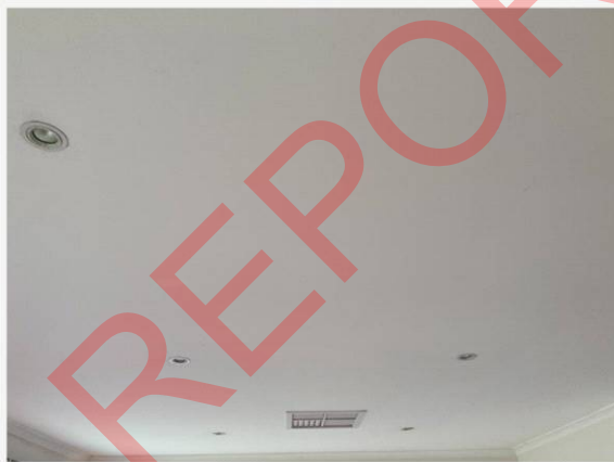
sagging/drop in ceiling noted example
