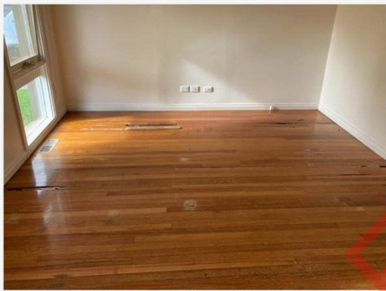
termite attack damage viewed to flooring
