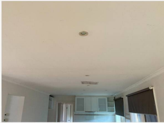
sagging/drop in ceiling noted example
