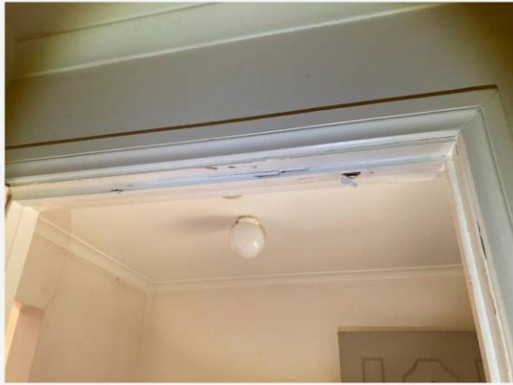
termite attack damage viewed to door jamb
