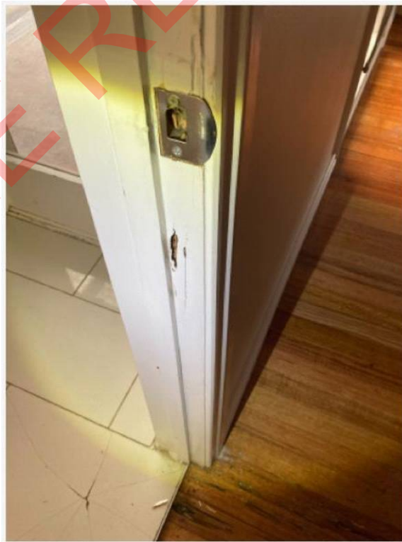
termite attack damage viewed to door jamb
