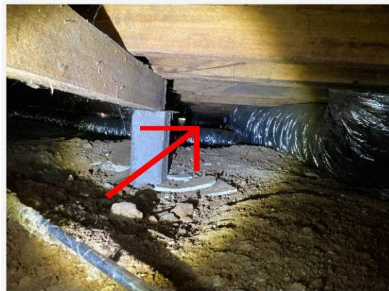
termite attack damage toward bathroom
