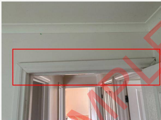
frame/jamb out of square
