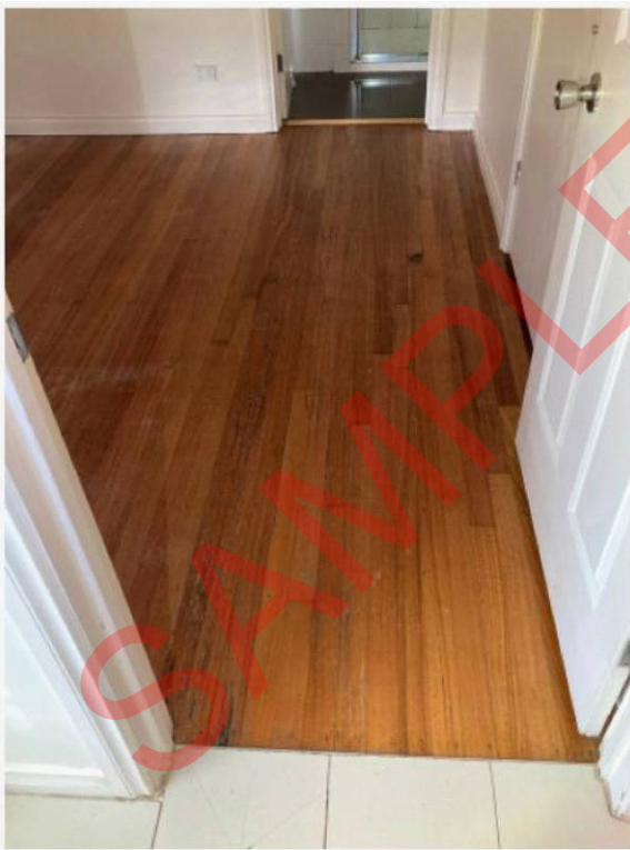
termite attack damage viewed to flooring
