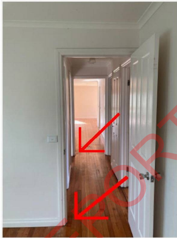
differential settlement/deviations noted
