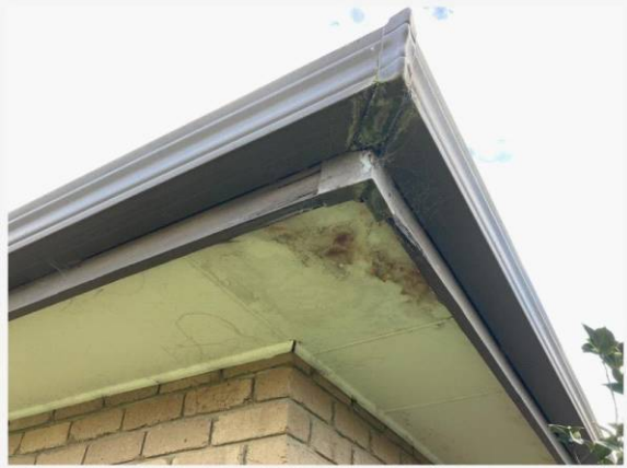
leak staining/damage noted to eaves
