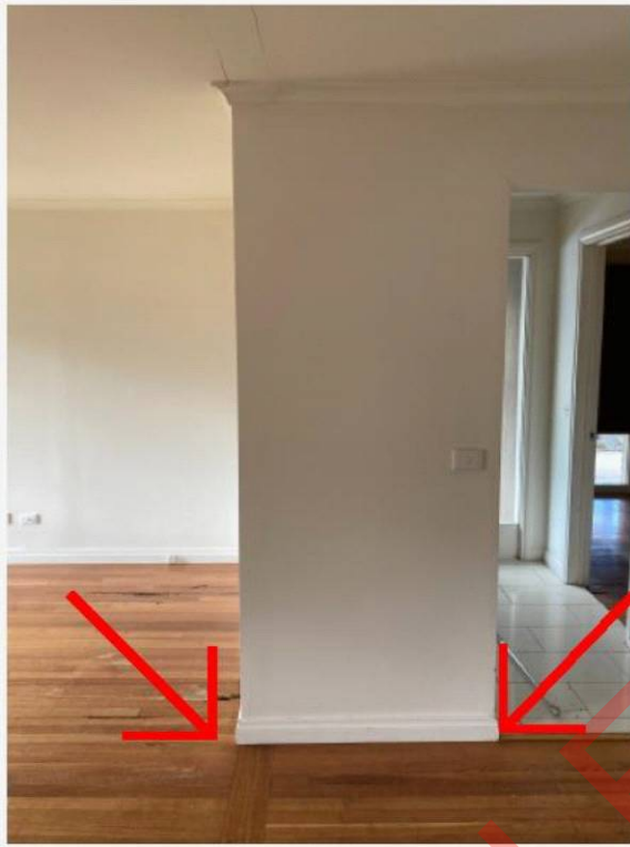
differential settlement/deviations noted
