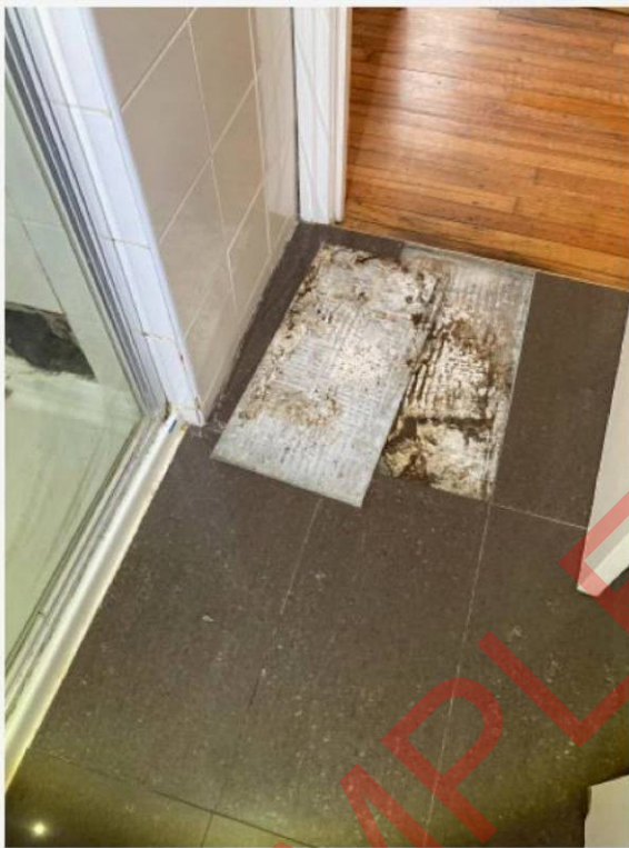
water spread / breach noted
