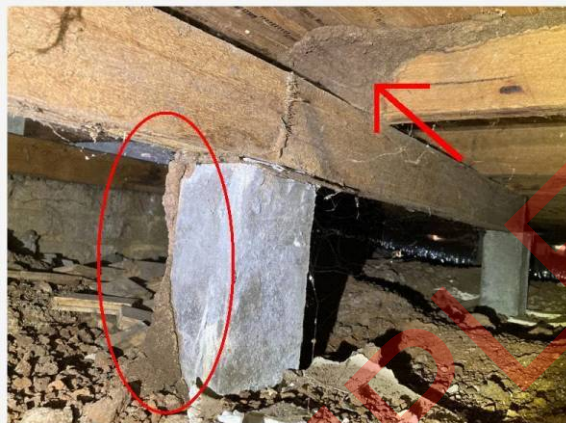
termite mud lead noted below entry/lounge
