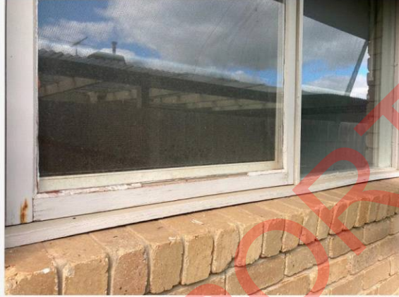
weathering/paint peel/minor decay noted
