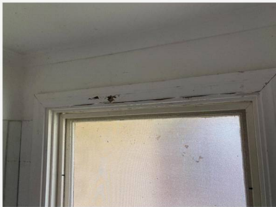
moisture damage viewed
