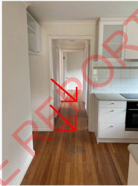
differential settlement/deviations noted
