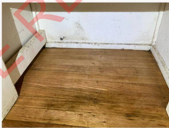
water spread / breach noted
