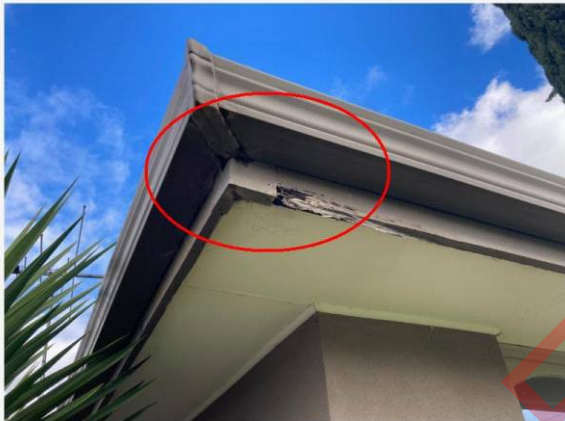
gutter leak causing timber decay example
