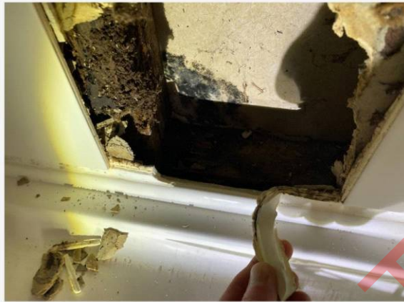
substrate not installed over tray flange
