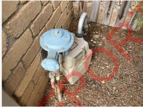
gas smell noted | have meter assessed
