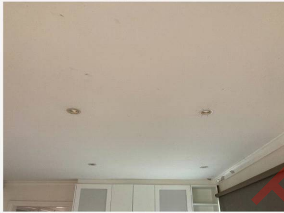
sagging/drop in ceiling noted example
