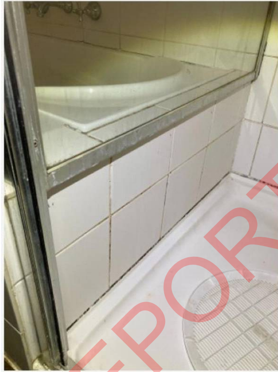
waterproofing defects visible
