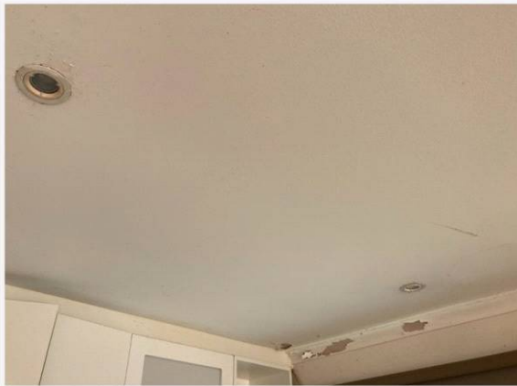
moisture/condensation damage viewed
