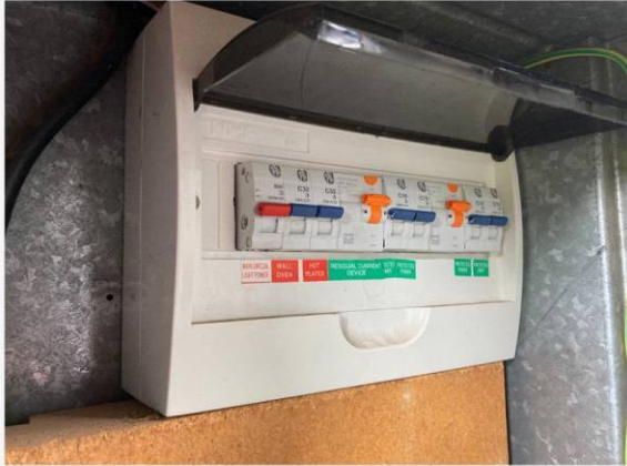
circuits appear OK | RCDs fitted
