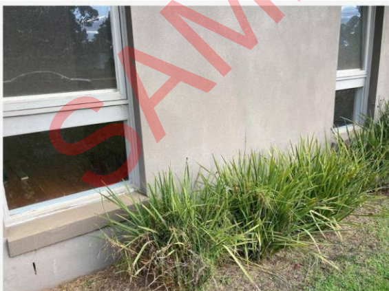
weathering/paint peel/minor decay noted
