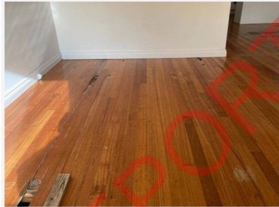
termite attack damage viewed to flooring
