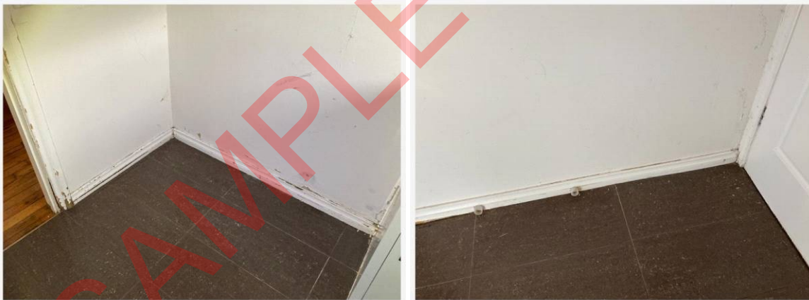
moisture/water/leak damage viewed
