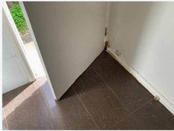
moisture/water/leak damage viewed
