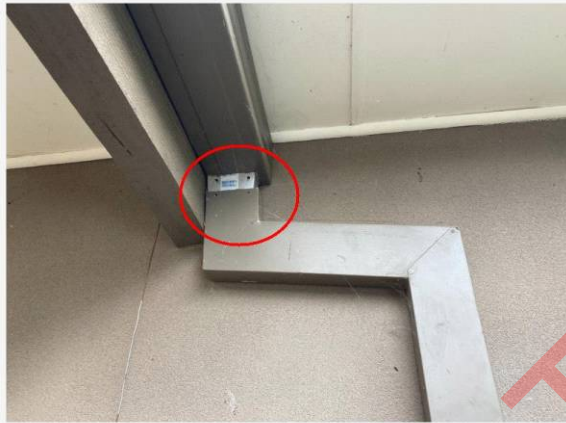
rework/secure DP to gutter pop
