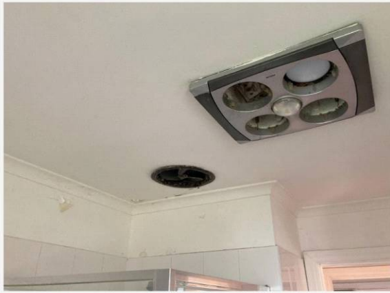
moisture damage viewed
