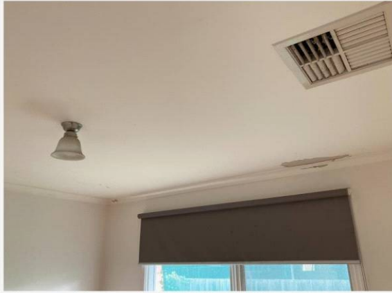
sagging/drop in ceiling noted example
