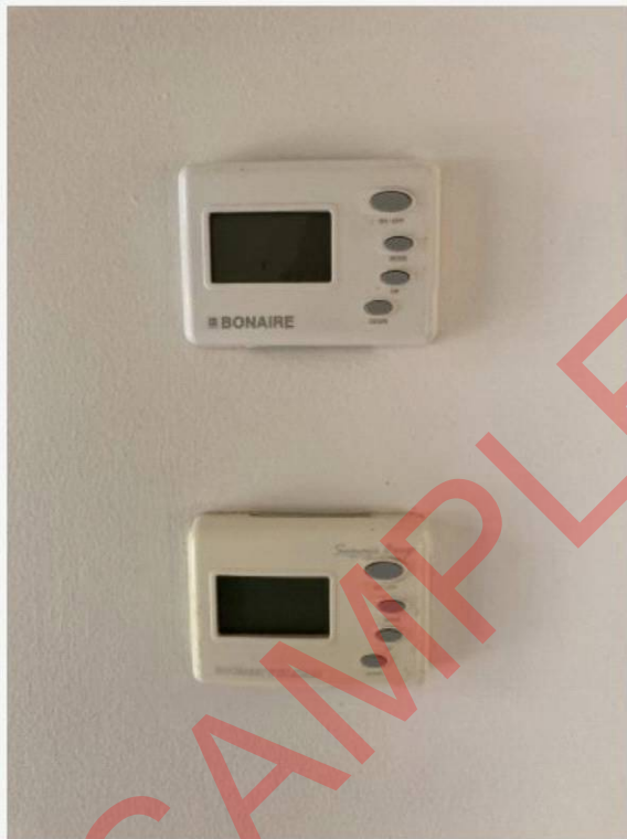
heating & cooling not tested on the day
