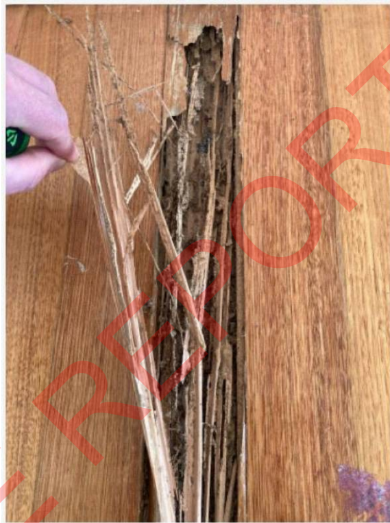
termite attack damage/workings viewed
