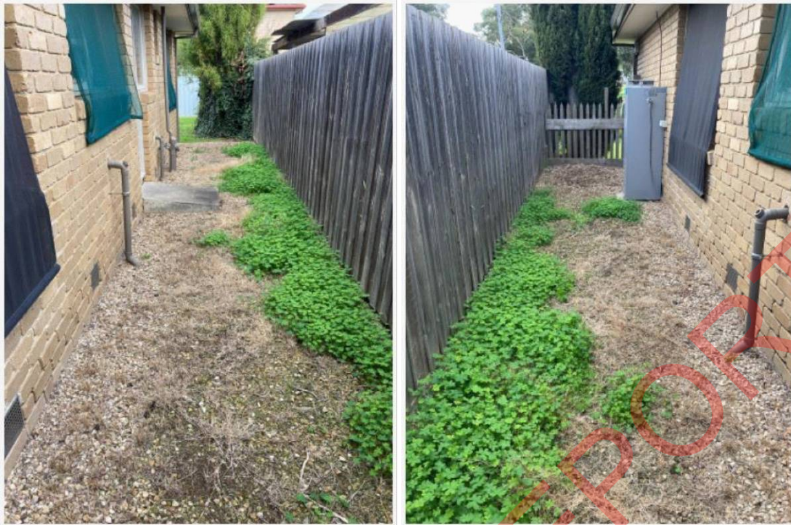
poor ground grading & drainage identified
